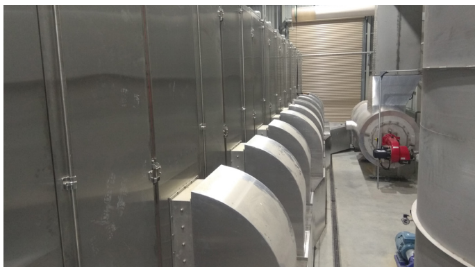
Burner (red) with combustion chamber and subsequent supply air fan for transporting the hot gas into the belt dryer
