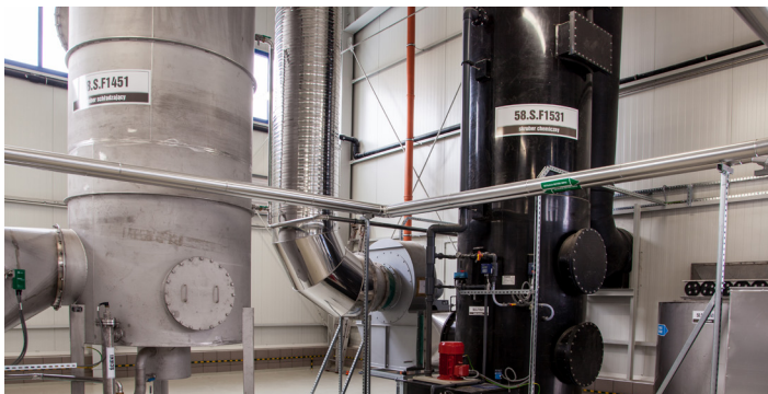
Wet and acid scrubber for exhaust gas
