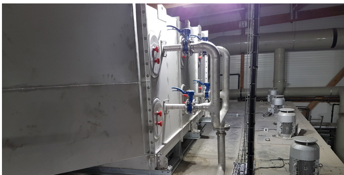
Circulation air fan and condensation
