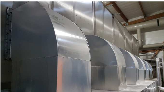
Belt dryer BD 3000/7 with exhaust air ducts
