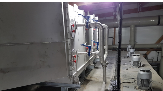
Circulation air fan and condensation
