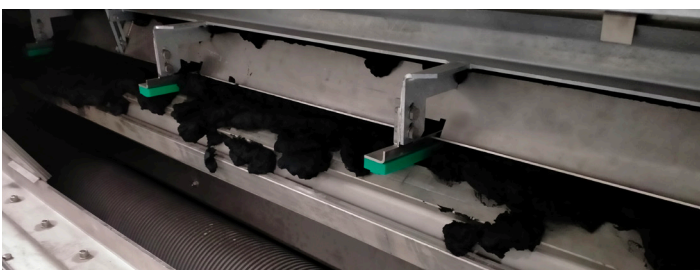
Dosing of back-mixed sewage sludge to Roller press
