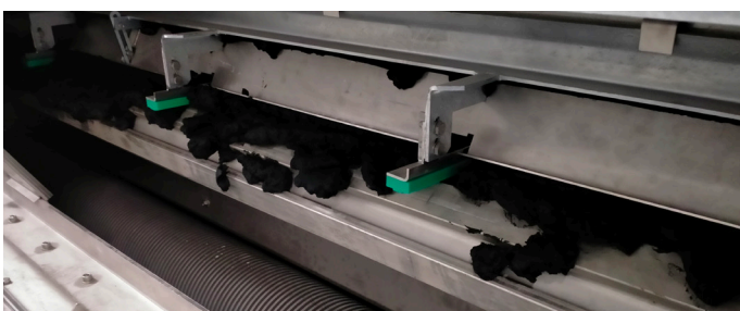
Dosing of back-mixed sewage sludge to Roller press
