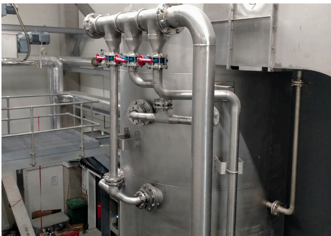
Preheating of the digested sludge in countercurrent column with humid warm exhaust air of the Belt Dryer
