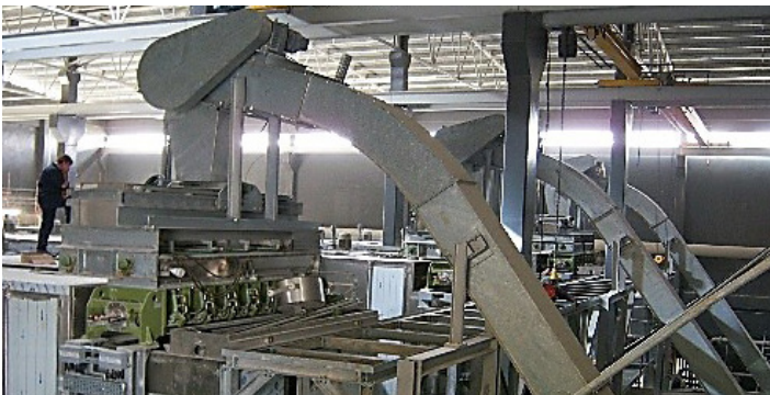
Trough chain conveyor for dewatered sewage sludge to the inlet unit (3x)
