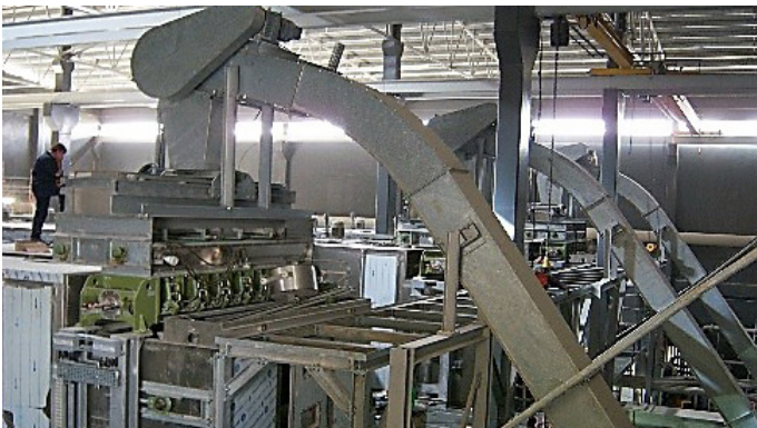
Trough chain conveyor for dewatered sewage sludge to the inlet unit (3x)
