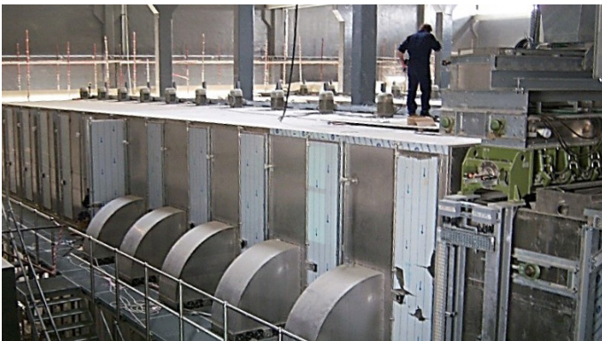
One line of the Belt Dryer BD 3000/12 with dryer inlet unit
