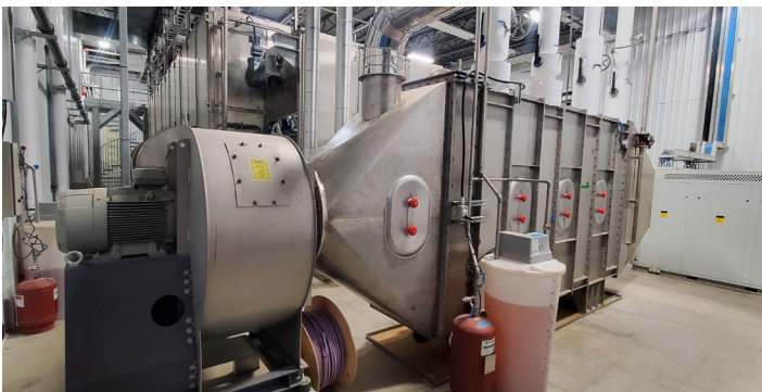
Supply air fan with heat exchanger and horizontal condenser
