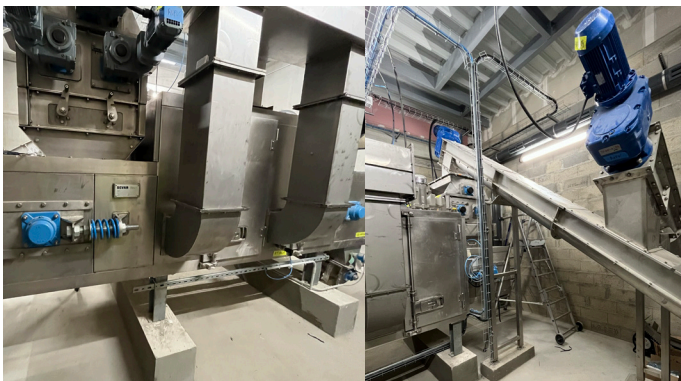
Left: Pilot dryer with feed unit and exhaust air ducts Right: Material feed via screw conveyor
