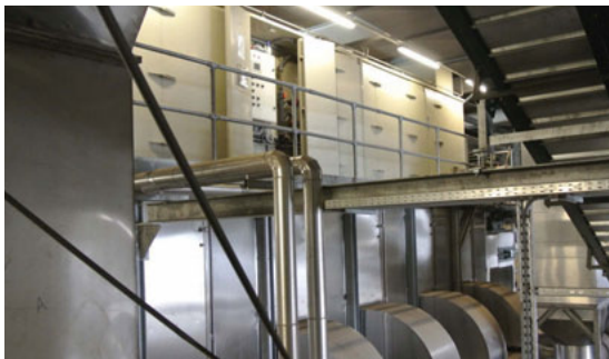
Chamber 1-3 of Belt Dryer BD 3000/5 with horizontal chemical scrubber
