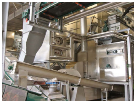
Combined inlet and outlet chamber with outlet screw conveyor
