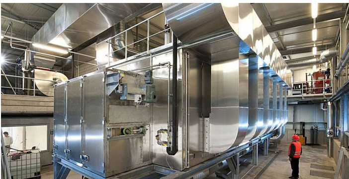
Belt Dryer BD 3000/6 with material return module and exhaust air ducts
