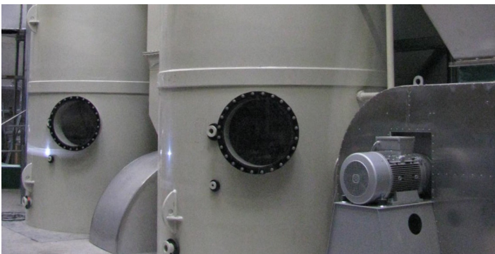
Chemical scrubbers (acidic & caustic)
